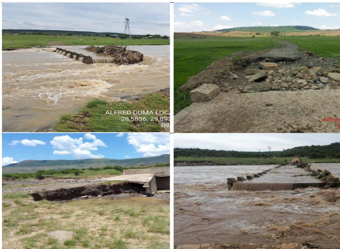
Figure 9: Damages on road infrastructure in the Alfred Duma Local Municipality (Source: Alfred Duma Local Municipality).
